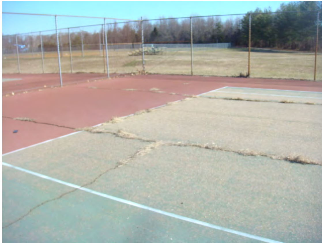
Tennis courts before repairs
